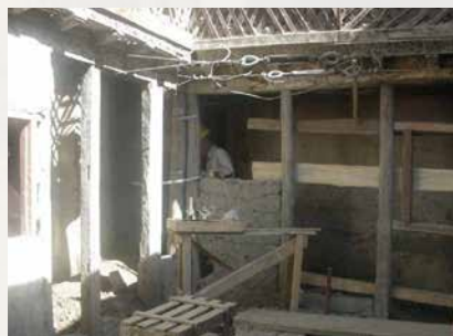
Fig 2: Decay of wooden elements
