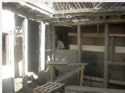
Fig 2: Decay of wooden elements
