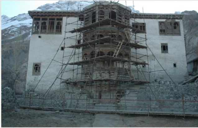
Fig 3: Above Pre conservation façade
